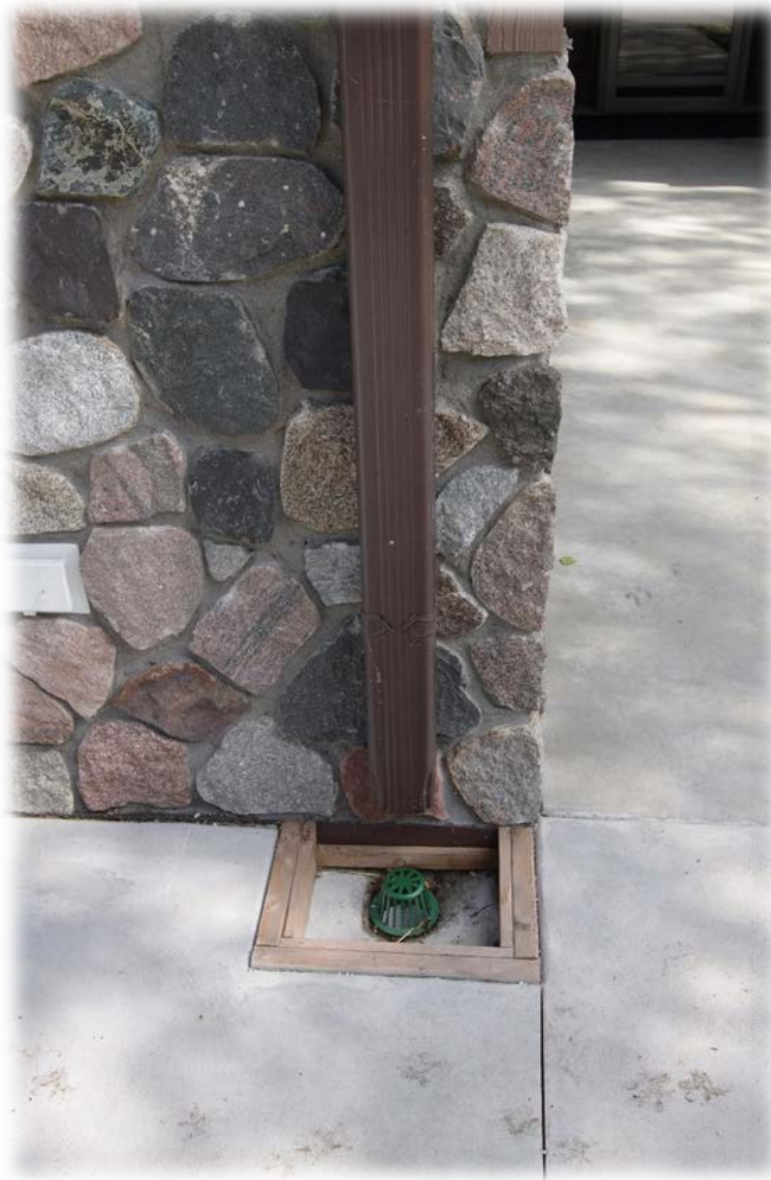
Figure 13. Sub-Surface Drains System
